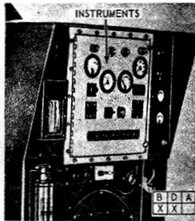
I. INSPECT FOR DAMAGE AND IMPROPER OPERATION.
